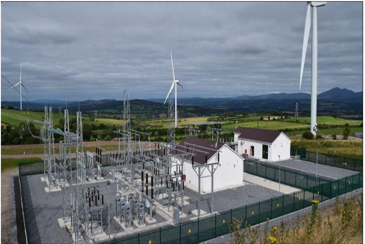
Plate 2.1: Example of a 110 kV AIS Substation
